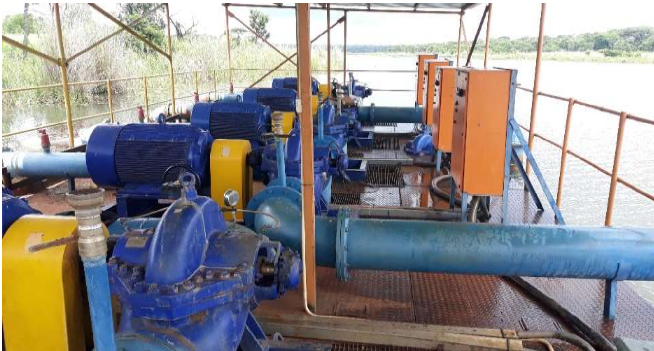
Figure 8: Floating Pump Station for Zambia Correctional Services at Musangashi Dam
